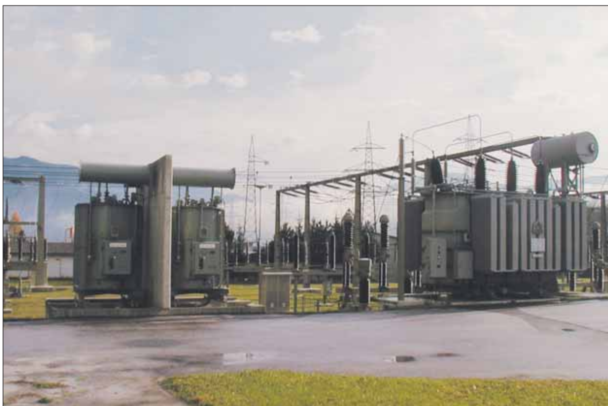
Fig. 1 110/20 kV Substation with arc suppression coils
